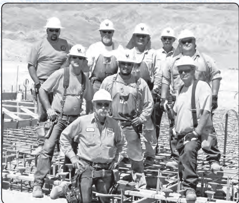
In the Owens Valley: Here's a DWP team building an irrigation distribution turnout station for water operations on Owens Lake. The team pictured is comprised of the concrete crews from Owens Lake Construction and the Mojave Construction Yards. They are, front row: Norm Harris, Building Repairer . Middle, from left: Jake Emory, Building Repairer ; Marin Parra, Reinforcing Steel Worker ; and Dave Borchert, Building Repairer . Back: James McMurry, Maintenance and Construction Helper ; Todd Emory, Building Repairer ; Ian Greer, Maintenance and Construction Helper ; Robert Turner, Construction and Maintenance Supervisor ; and Jerry Ross, Maintenance and Construction Helper . Special thanks to Larry Patrich, Construction and Maintenance Supervisor, DWP, Club Member, for sending us the photo.
