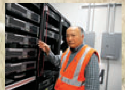
Michael Lee, Electrical Engineering Associate, demonstrates the sever room.
