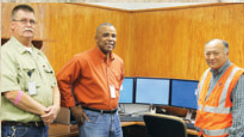
From left: Larry Patrich, Labor Supervisor; David Neal, Operations Manager; and Michael Lee, Electrical Engineering Associate, in the under-construction SCADA (Supervisory Control and Data Acquisition) room, where many of the dust mitigation systems are monitored. By custom-building this room using their own staff's expertise, the Owens Lake team saved the DWP $90,000.
