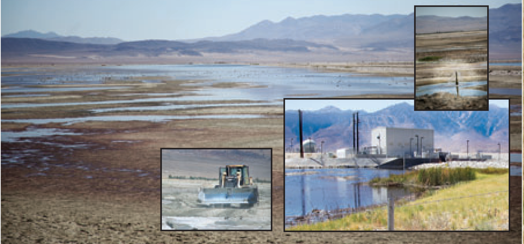
A dozer clears a flood channel (left); the pumping station at the end of the Lower Owens River (middle); a bubbler is used to distribute the water (right).
