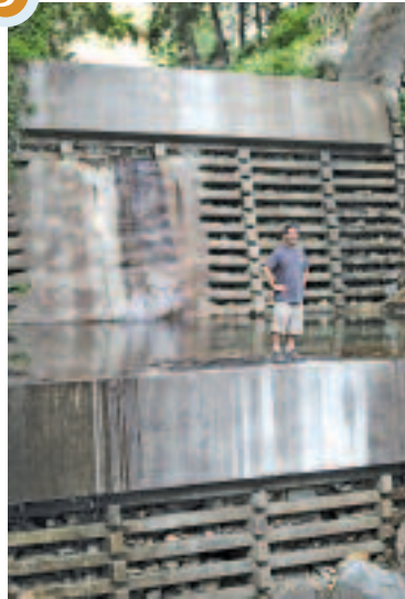
These are the erosion dams built to control water flow, I believe.
