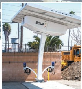
Some of the 10 new BEAM electric chargers for StreetsLA's yards.
