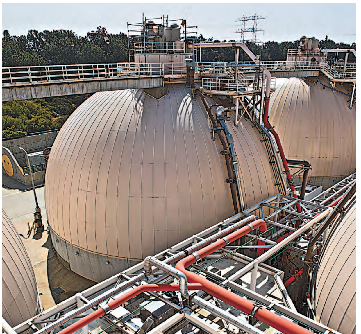
The large digesters at the Hyperion Water Reclamation Plant.
