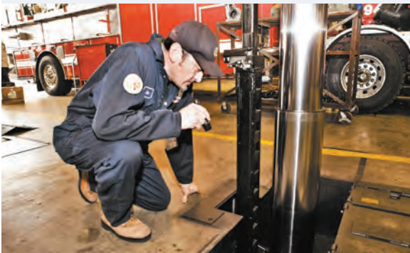
From April 2017: Alex Garcia , Elevator Mechanic, General Services, 17 years of City service, inspects a lift at the Lincoln Heights LAFD Supply and Maintenance facility.
