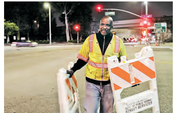
With the fans safely on their way home, Richard collects the barricades and calls it a night. Job well done!
