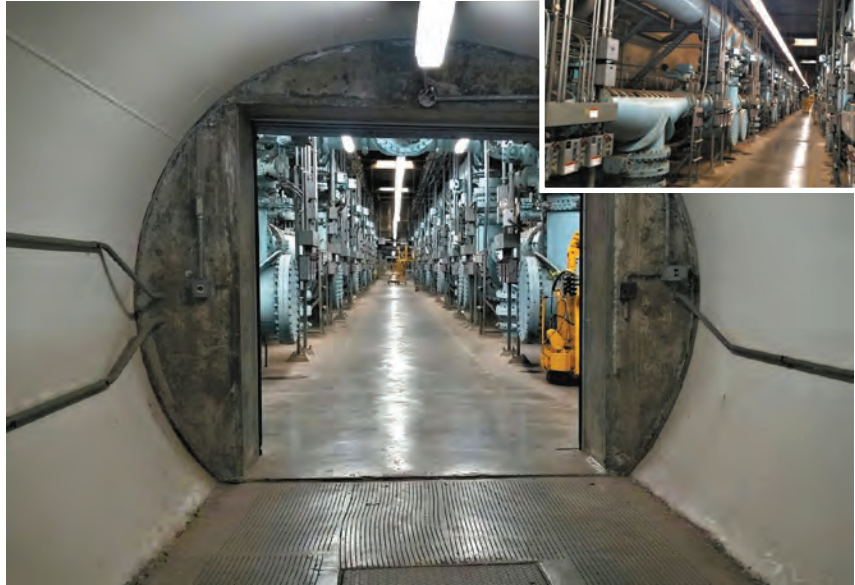
"Looking at the vast network of pipes under the aqueduct filtration plant, Sylmar. This photo was taken from the service entrance, which was constructed from 120-inch pipe used for the reservoir outlet."
