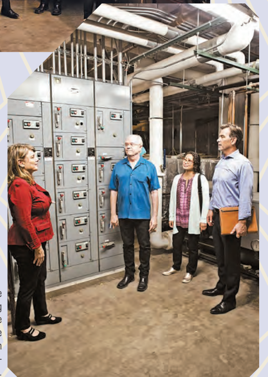
RIGHT: The City paid for the replacement of the theater's heating and air conditioning systems. The air circulation system uses the same grated vents in the floor of the main theater that the original construction used in the 1930s.
