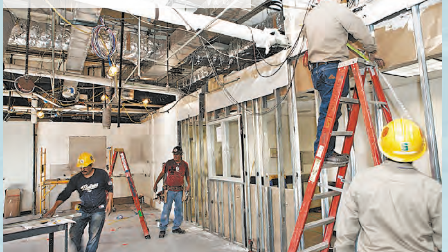
Construction Forces workers transform a Piper Tech storeroom into a bright clerical workspace for the LAPD's SID DNA unit.
