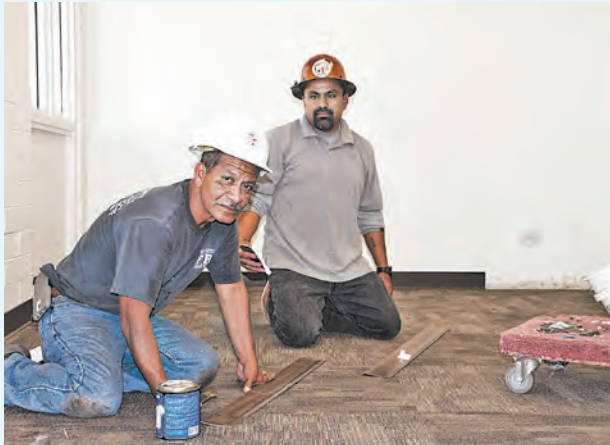
Installing carpet and floorboards are (from left) Liborio Damian, Carpet Layer, 12 years of City service; and Luis Cuevas, City Crafting Assistant, 8 years. Not pictured: Jerry Jimenez, Carpenter, 2 years.
