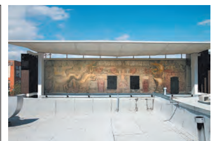
The famed mural, on a wall that was reinforced and sealed from behind by Construction Forces.
