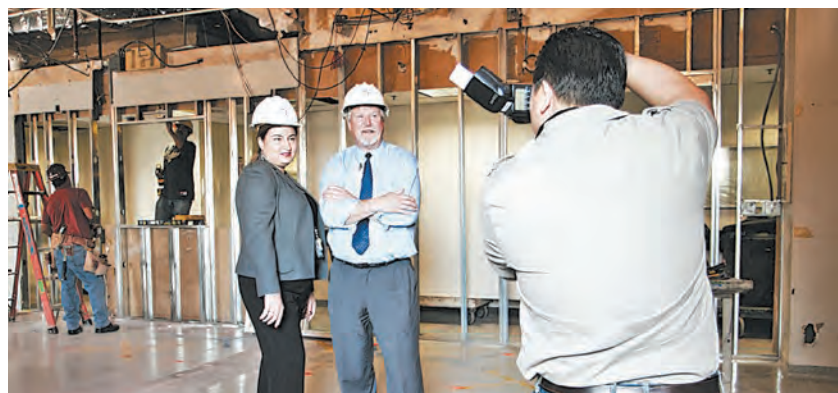
The Club's Summy Lam (right) photographs Construction Forces' Rose Karagezyan and Nick Pendorf at the under-construction LAPD SID DNA space at Piper Tech.
