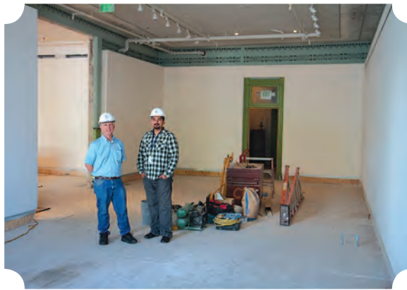
The inside of the Sepulveda Building during construction, June 2012. Pictured are (from left) Eric Hess, Sr. Construction Inspector, Public Works/Contract Administration, and Javier Gonzalez, Construction Manager, Public Works/Engineering.
