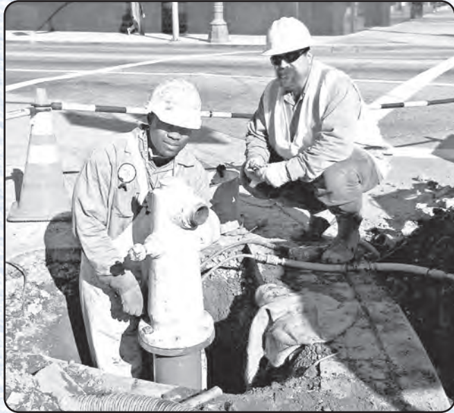
Repairing a fire hydrant at Second and Spring Street downtown are, from left: Tommy Gibbs , Water Utility Worker, 14 years of City service; and Vernon Chesterton , Sr. Water Utility Worker, 8 years.
