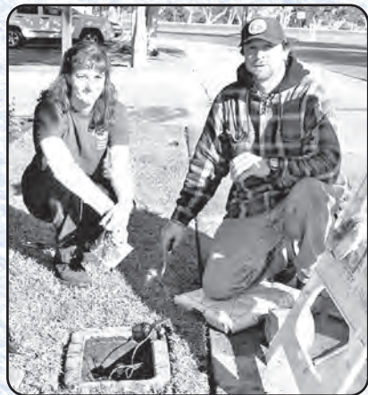
Here's a photo of Rec and Parks employees working on an irrigation system near the Cabrillo Marine Aquarium in San Pedro. From left: Traci Rubner , Sr. Gardner, 9 years of City service; and Frank Holmes , Irrigation Specialist, 1 year.
