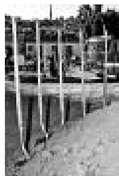
Shovels line the mound of dirt that will begin the building process as the new station's Engine 78 is parked in the background.
