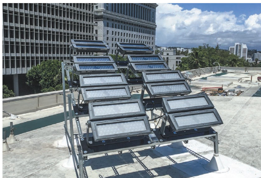
Some of the lighting fixtures used to illuminate City Hall.
