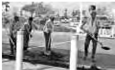
From left: Connie Gomez, Miguel De La Parra, Gary Ramirez and Paul Flowers of the LA/Ontario International Airport Field Crew assist with the repaving of the terminal roadway.
