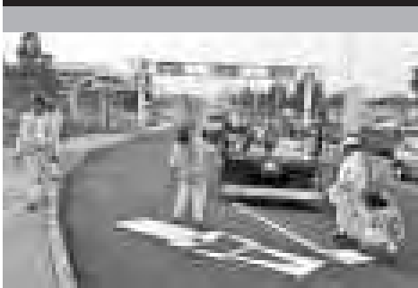
After placing templates on the ground, Ontario field paint crew members (from left) Nestor and Ricardo Mediano stand by while Larry Hartnet, Antonio Aleman and Brian Heath paint surface traffic markings.
